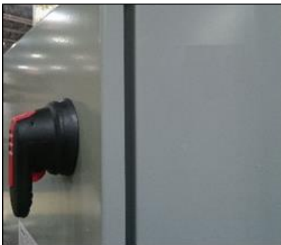
Figure 1. Disconnect Switch Junction Box
