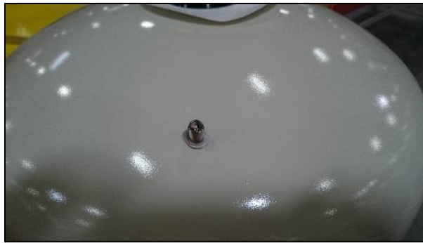
Figure 3. Top of Expansion Tank
