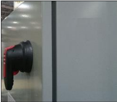
Figure 2. Disconnect Switch Junction Box
