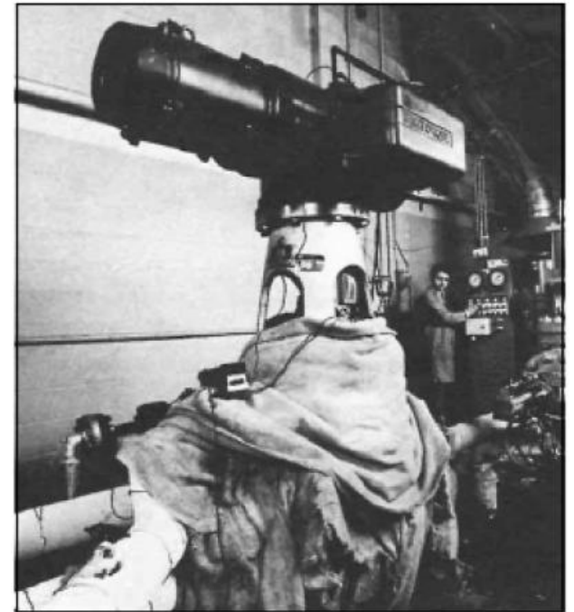
Figure 2: A size 16 (400mm) class 1500 Flowserve-Edward Equiwedge gate valve with a Flowserve-Limitorque actuator undergoes hot-functional testing.
