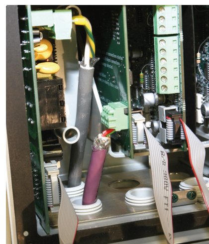
FIGURE 12-5. Complete Profibus board installation with ribbon cable attached.
